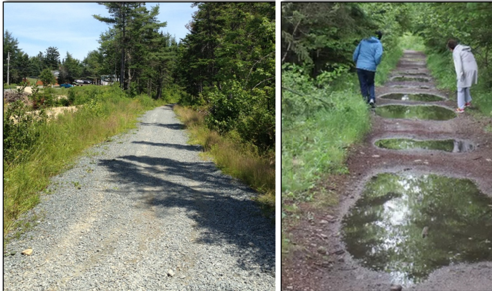
Figure 2-9: Blueberry Run existing conditions. Poor compaction (left) and ponding (right)
