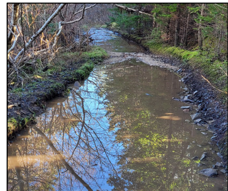
Photo 2-2: Abandoned CN Railway Ponding
